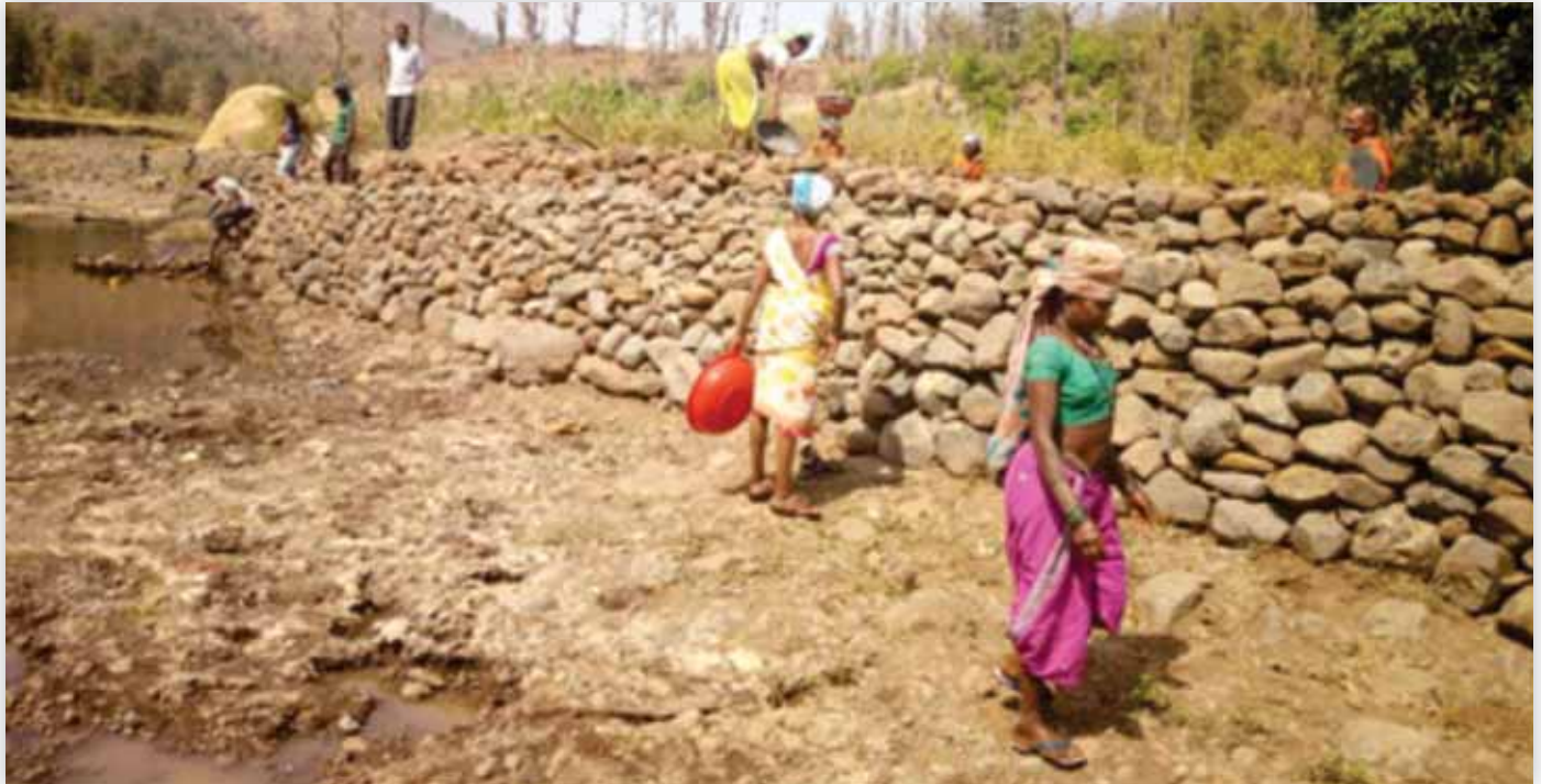
This small looking stream becomes powerful in monsoon & erodes farms on the banks. Hence a tall bandhpala is built to protect the farms. Such a stone wall will prevent soil erosion & will prevent stream water from entering farm.
